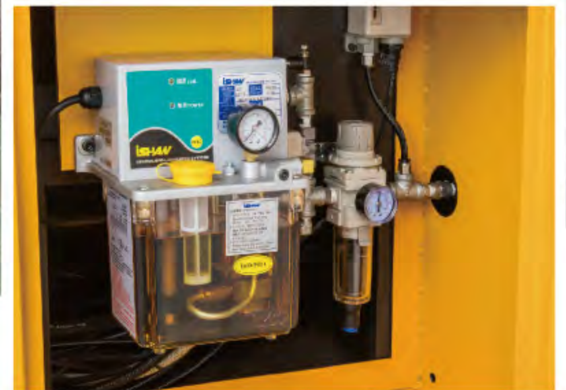
Automatic lubrication unit.
